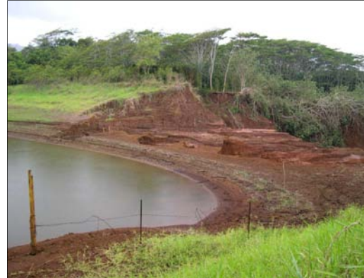
Figure 2 - Breach as seen from the right abutment
