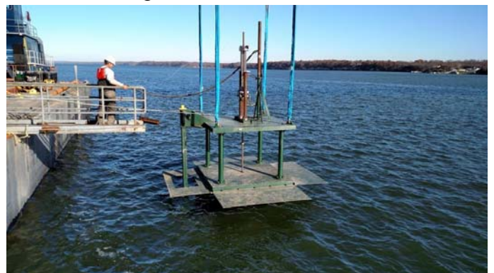
Figure 1: Lowering the seafloor direct push system into the river with a large crane
